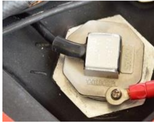
(Fig. 9) Showing grounding wire attached to the Electronic Level Sensor.
